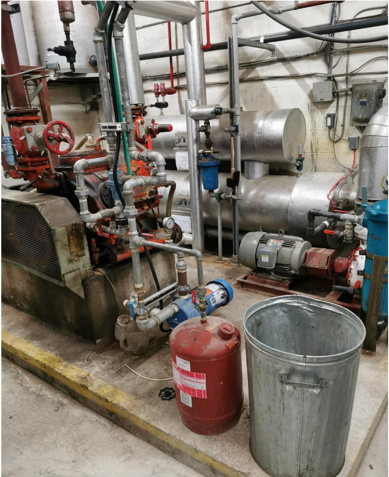
Figure 5: Humboldt Curling Rink Refrigeration Plant
