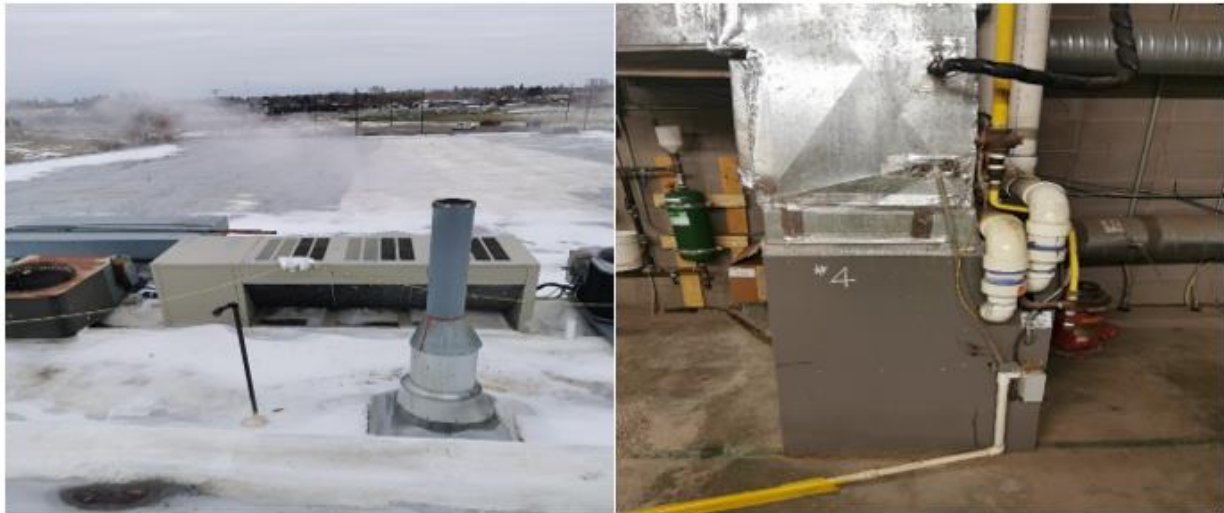
Figure 20: Humboldt Community Room HVAC
