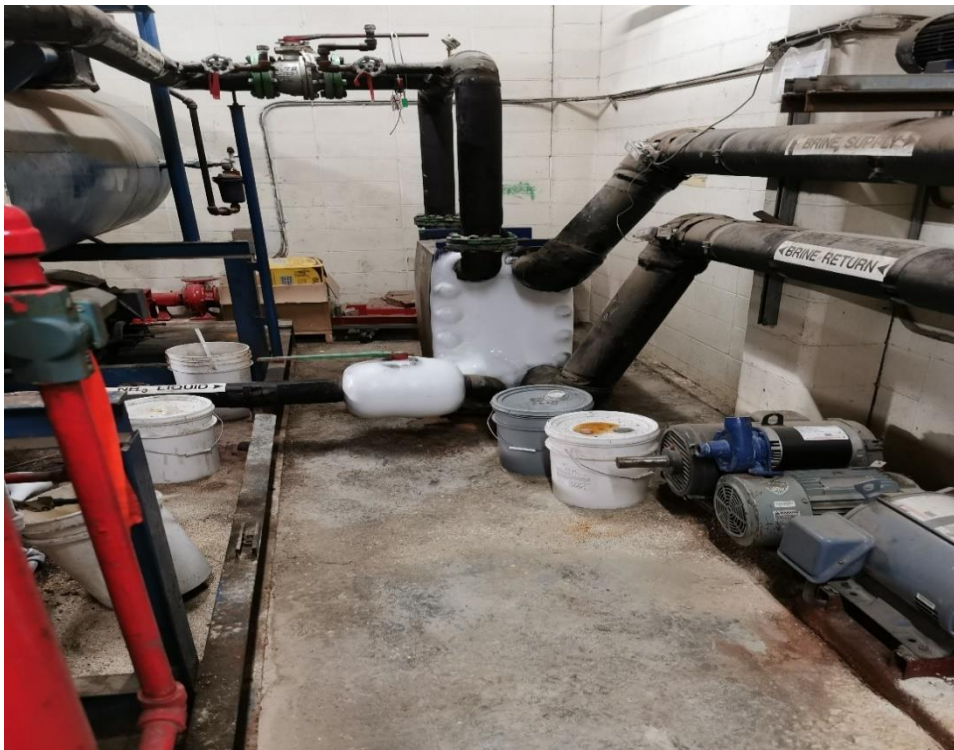
Figure 3: Humboldt Arena Chiller
