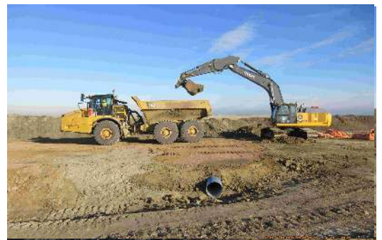
Figure 1: EllisDon installing a culvert in the south end of the project site. Courtesy of Howie McInnes
