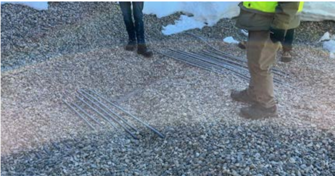
Figure 6: Aeration Pipes in SAGR Cell Bottom - March 5, 2025
