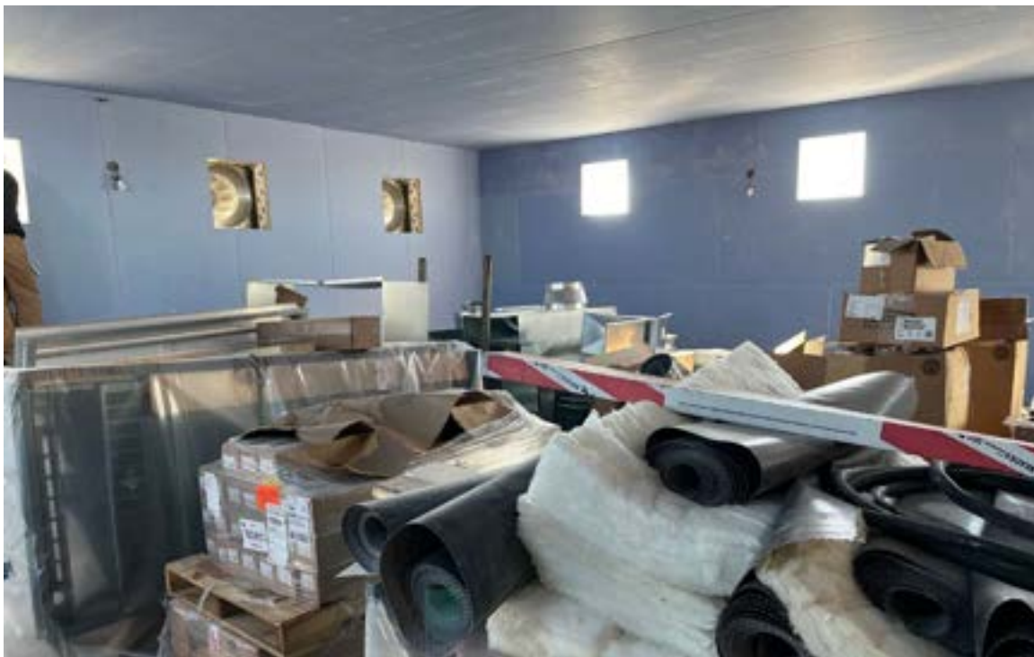
Figure 4: Blower Room - Operations Building – March 5, 2025
